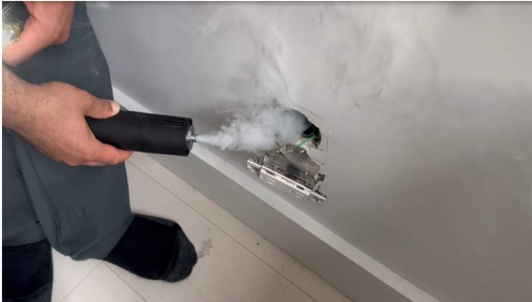
Figure 1 Apartment 6B Smoke Exfiltration
