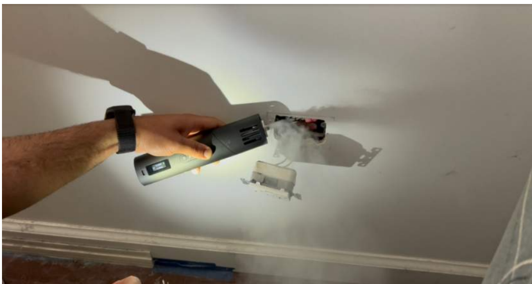
Figure 2 Apartment 6A-N Smoke Infiltration
