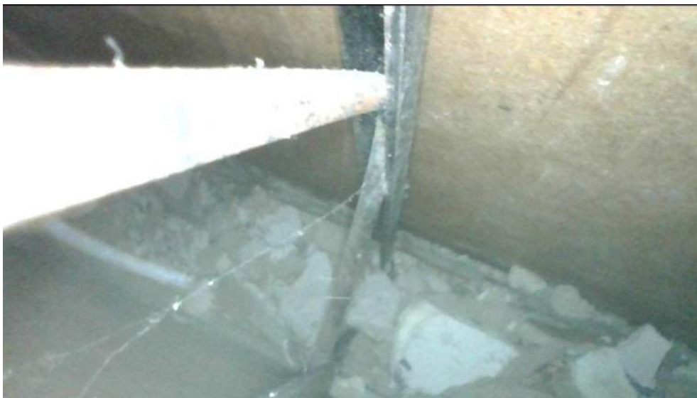
Figure 4 Demising Wall Borescope Image
